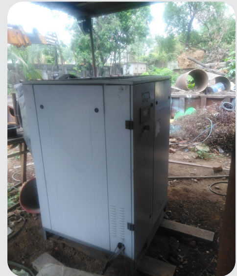
Figure 1: Existing fixed speed air compressor
